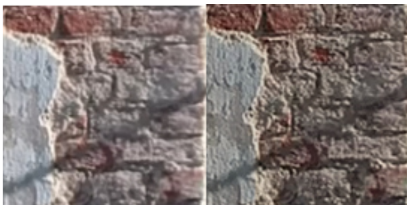
Figure 7. Detail of the façade degradation (highlighted in green in the Figure 5) for the Orthophoto generated with Pix4D (left) and MicMac (right).
