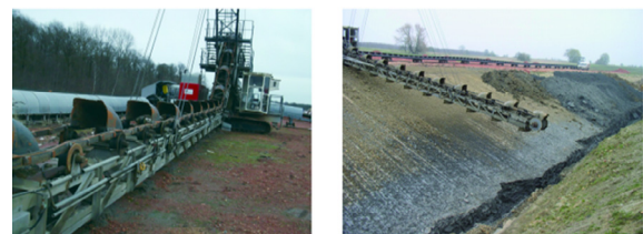
(a) Chain bucket excavator operating onsite, front view (b) Chain bucket excavator in operation in silty soil, lateral view
