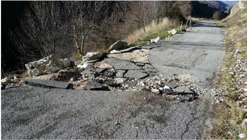
Figure 4.58. Damage to road from 1-2.5 m boulder impacts from rockfall between sites 9a and 9b.
