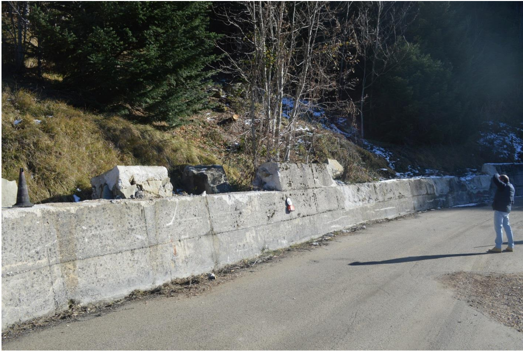
Figure 4.52. Damaged segmented concrete block retaining wall at roadway. Blocks that fell on road have been removed by local officials prior to visit from GEER team.
