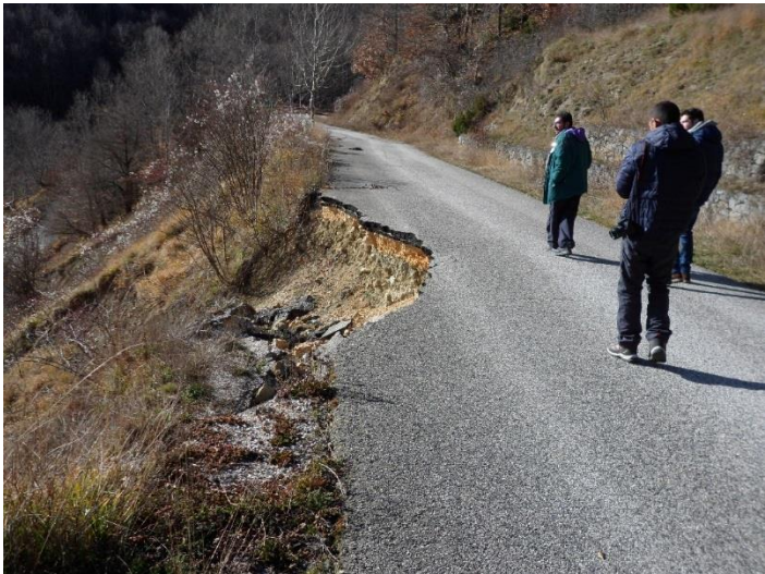
Figure 4.93. A slide observed on the fill slope.
