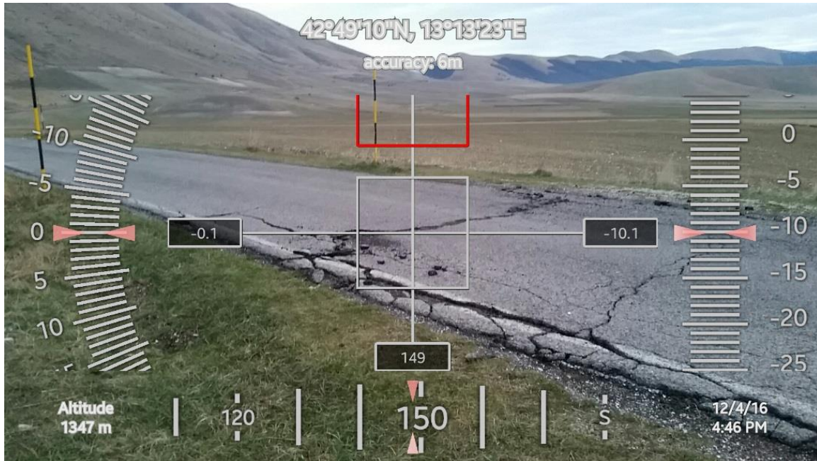
Figure 2.20. Secondary fault offset across a road on the Piano Grande at the base of the Mt. Vettore Massif. August 2016 event offset of 0cm. October 2016 event offset of 7 to 18 cm.
