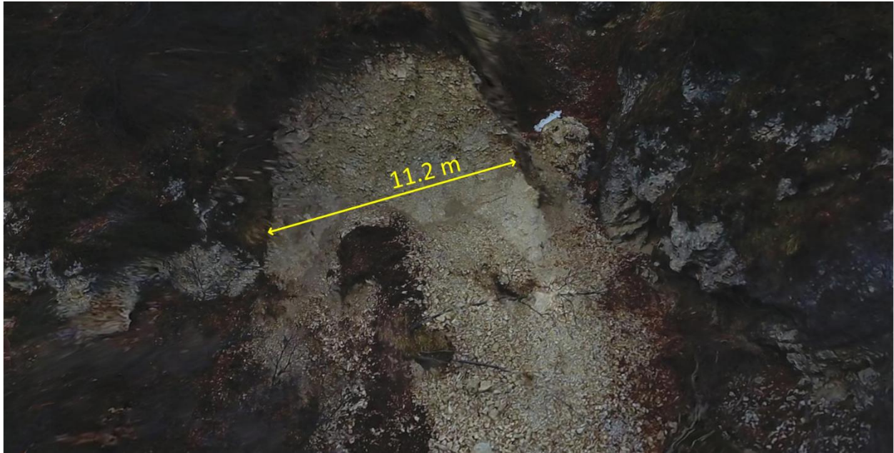
Figure 4.42. 3D model of the source of the Valle di Panico rockfall, located 90 meters above the mountain road.
