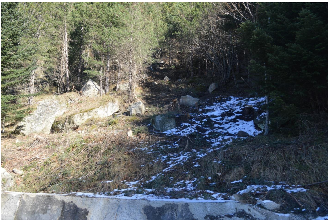
Figure 4.53. View upslope of damaged retaining wall, boulder fragments and runout chute from road at rockfall site near Crognaleto village.
