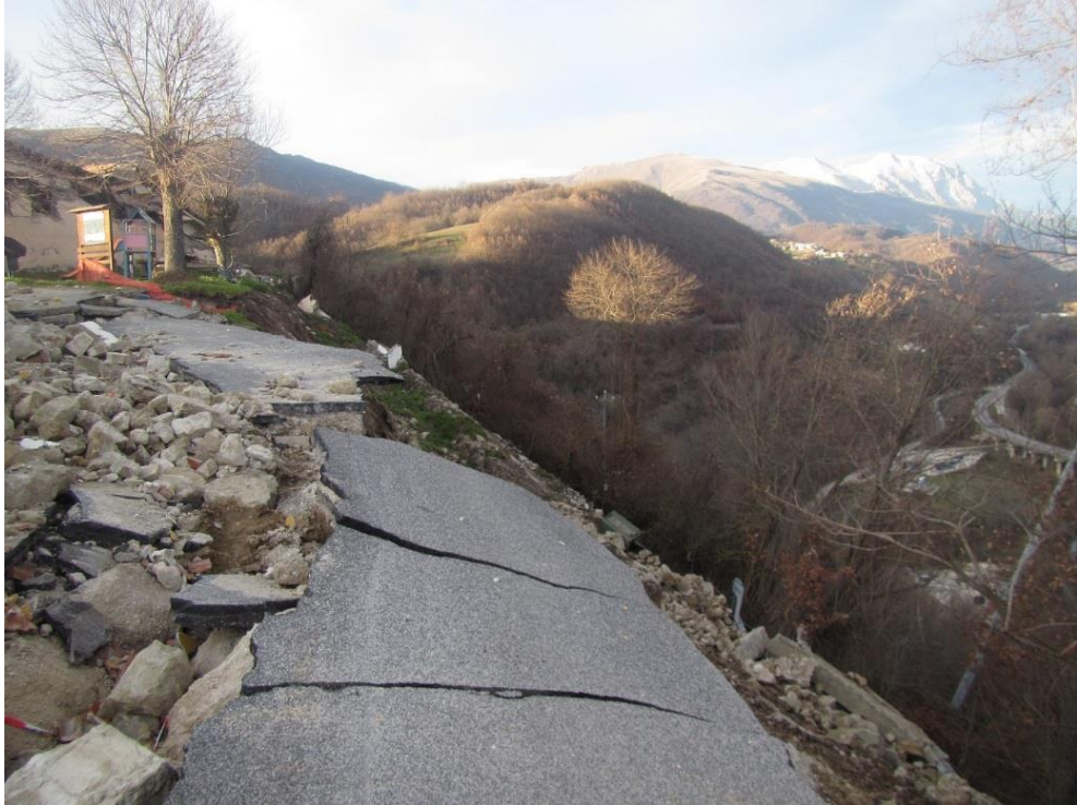
Figure 4.30. Failure of retaining wall due to shallow landslide (Point 4a, looking towards north).
