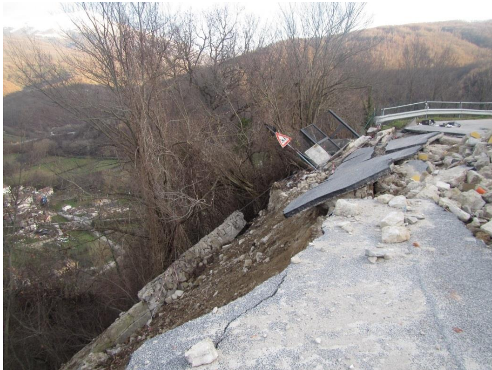
Figure 4.31. Failure of retaining wall due to shallow landslide (Point 4a, looking towards south).
