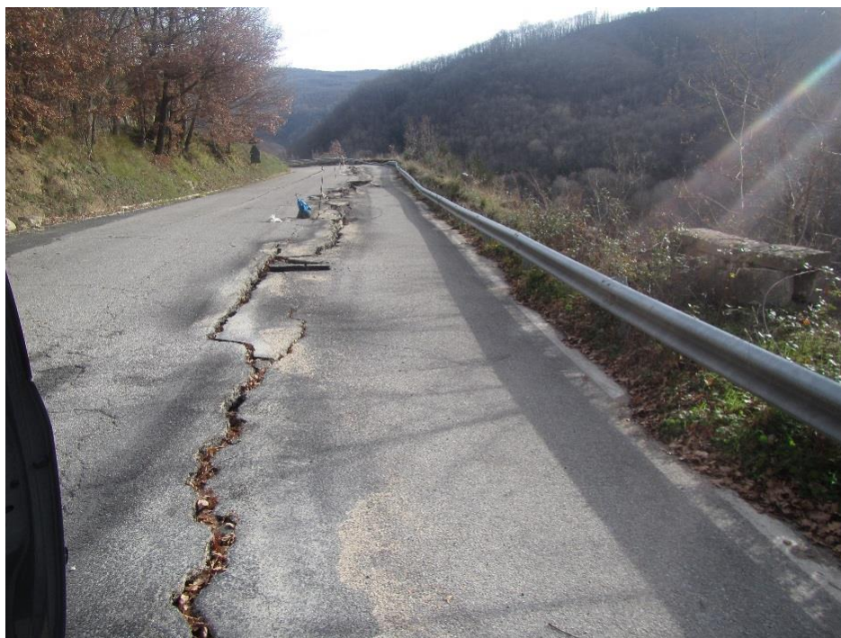
Figure 4.17. Road damage induced by slight rotation of the underlying retaining wall and/or settlement of the retaining wall backfill.
