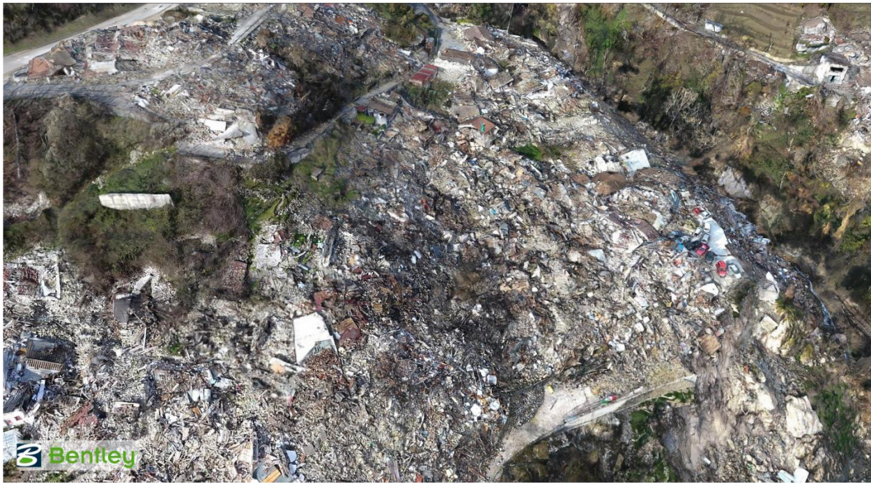
Figure 4.14. 3D SfM model of main damaged building area overlying talus deposits (Location 3a).
