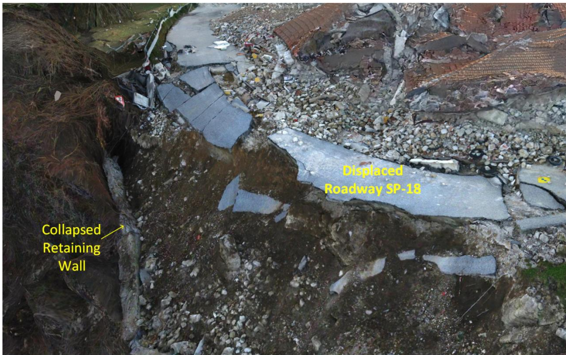
Figure 4.33. 3D model screenshot of the destroyed roadway Frazione Fonte del Campo (i.e., SP-18).
