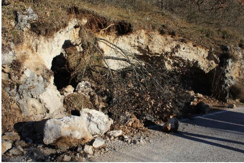
Figure 4.75. Rockfalls with boulders on the road.
