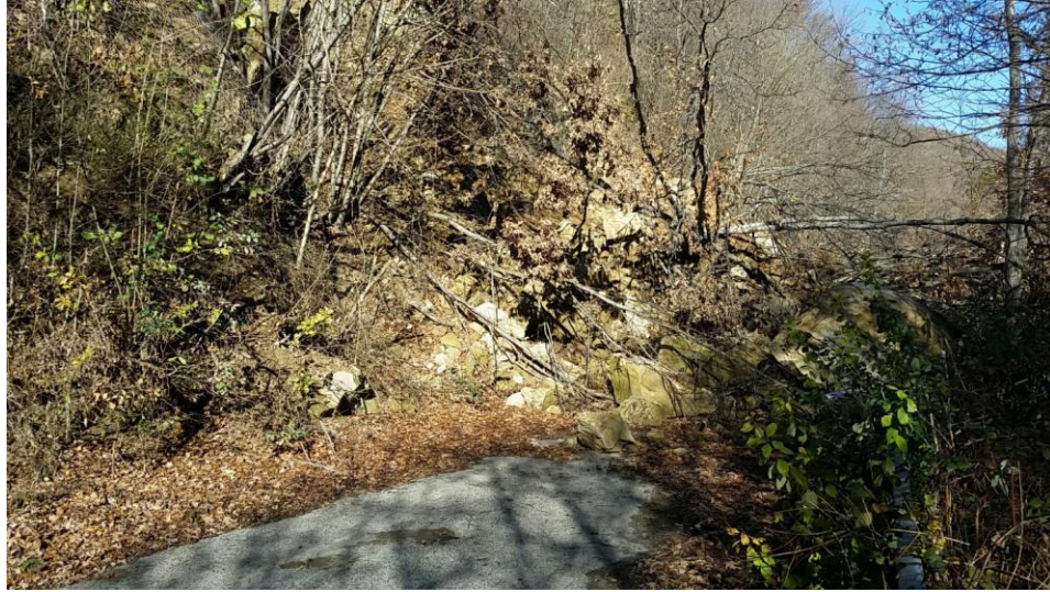
Figure 4.101. Landslide debris covering the roadway. Boulders range in size up to 2 meters. Also pictured is rockfall netting used by local officials for minor rockfall control on the slope.
