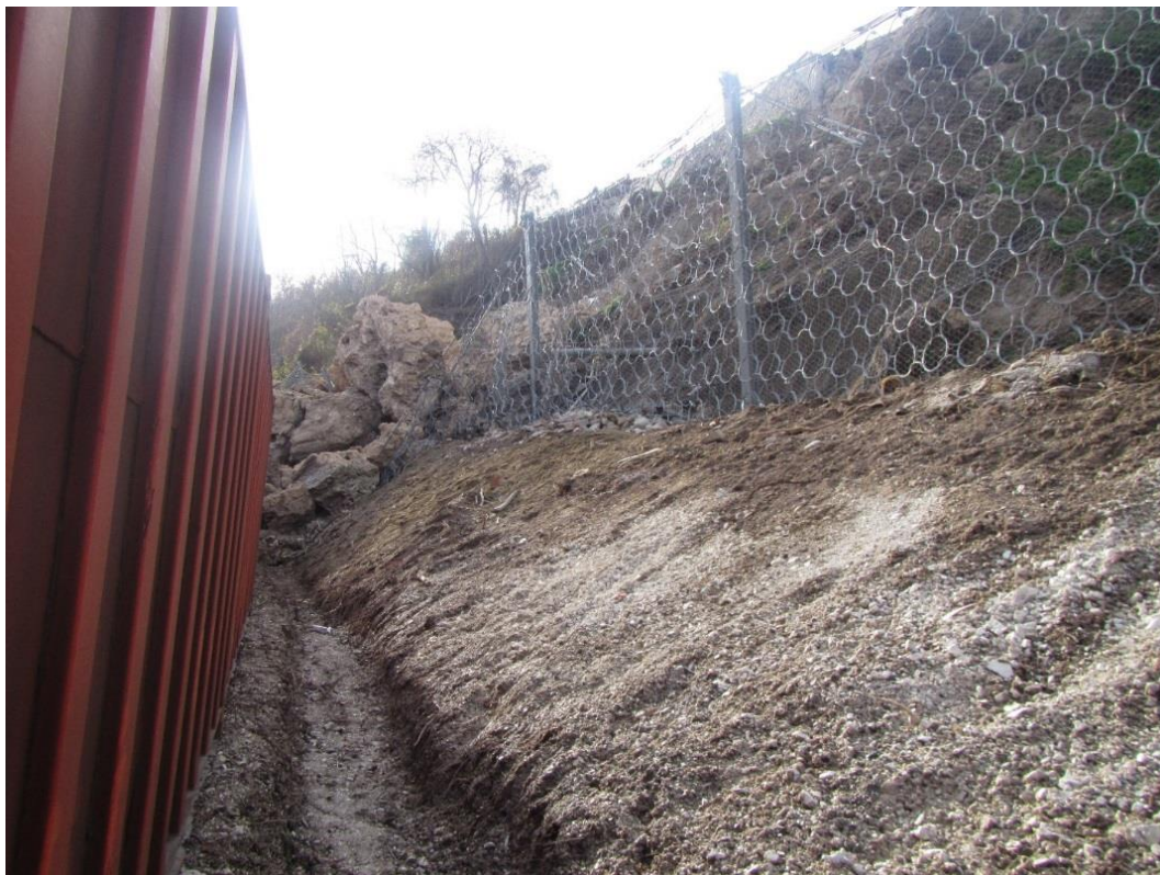
Figure 4.19. View of damaged rockfall netting caused by loose debris material from the landslide above Strada Statale No. 4 (Location 3d).
