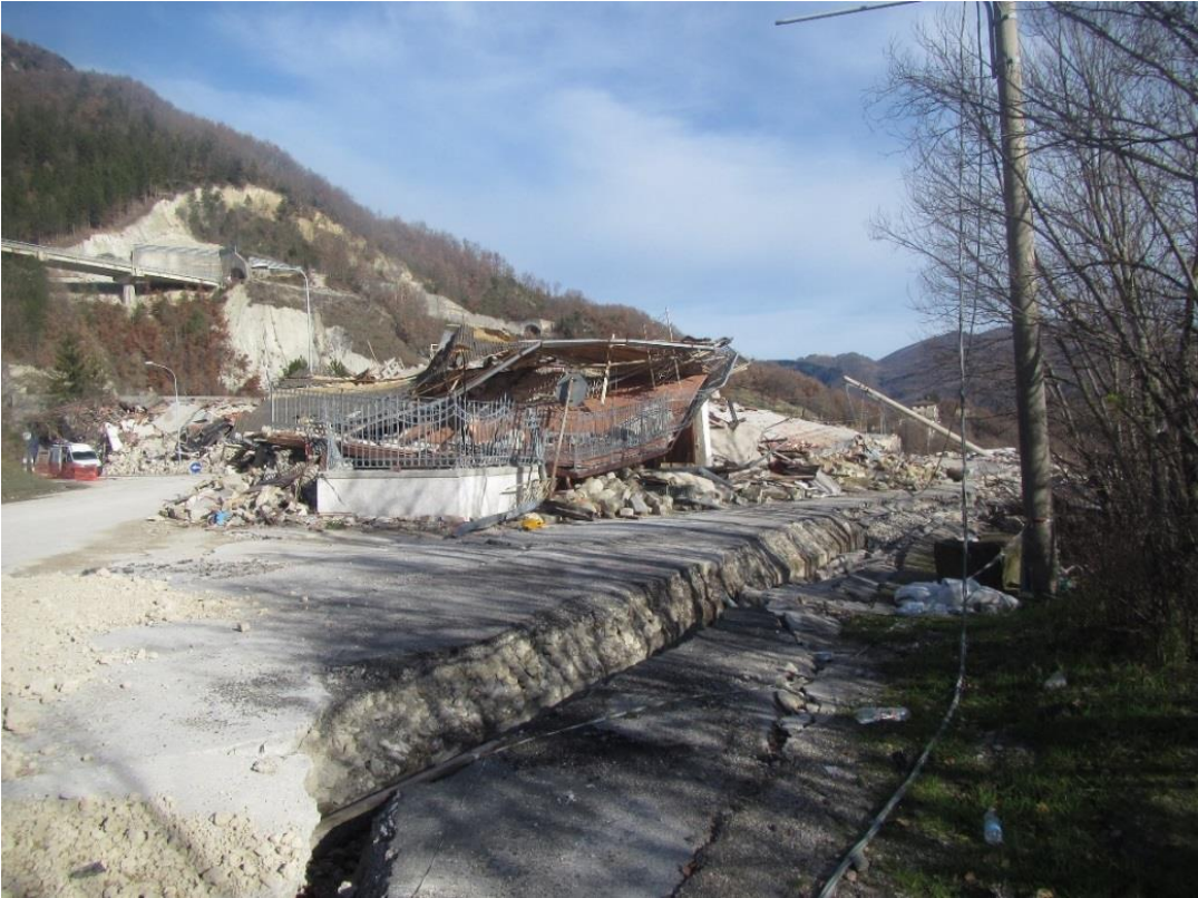
Figure 4.16. Pavement and road base damage induced by underlying stability failure of fill material (Location 3c).
