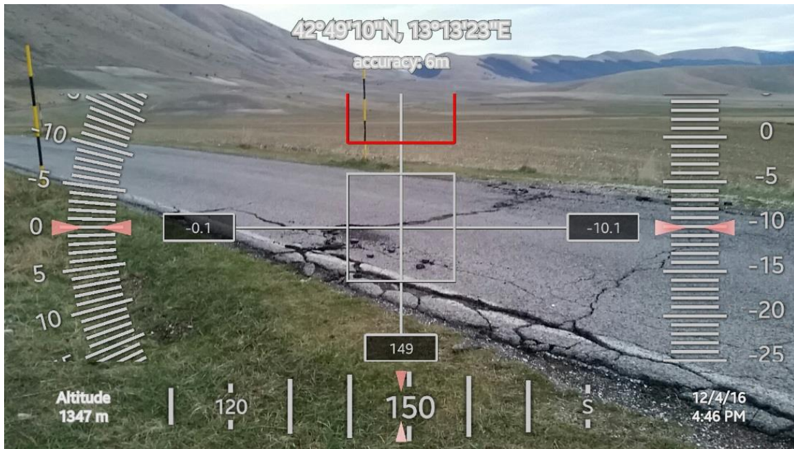
Figure 2.20. Secondary fault offset across a road on the Piano Grande at the base of the Mt. Vettore Massif. August 2016 event offset of 0cm. October 2016 event offset of 7 to 18 cm.
