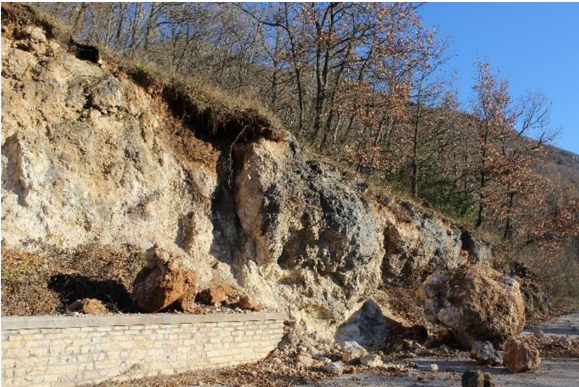
Figure 4.74. Rockfalls with boulders on the road.
