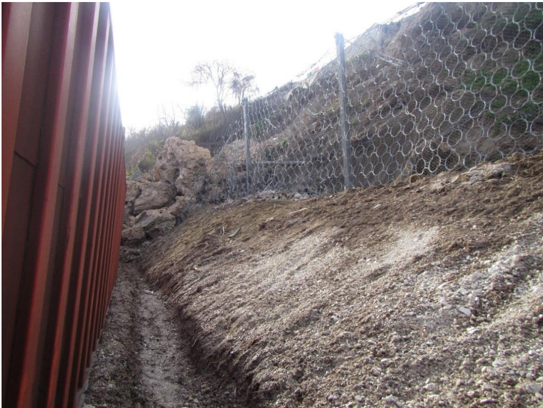
Figure 4.19. View of damaged rockfall netting caused by loose debris material from the landslide above Strada Statale No. 4 (Location 3d).
