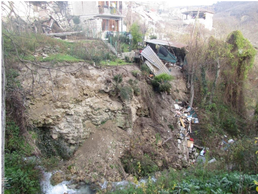
Figure 4.20. Failure of steepened talus gully wall material and crest area above (Location 3e).
