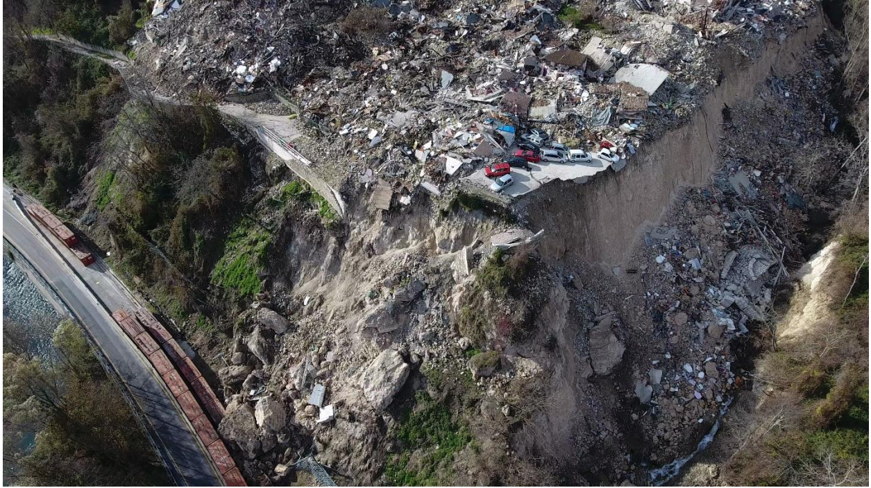
Figure 4.18. Aerial photograph of landslide impacting Strada Statale No. 4 below Pescara del Tronto (Location 3d).
