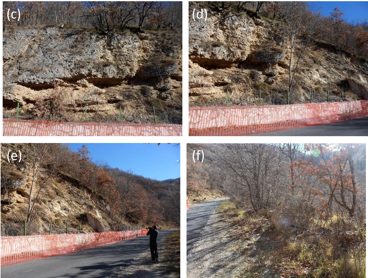
Figure 4.89. Failure in calcareous breccia between Cittareale and Norcia along the SP746: from (a) to (e) view of the all facade; (f) rockfall on the road.
