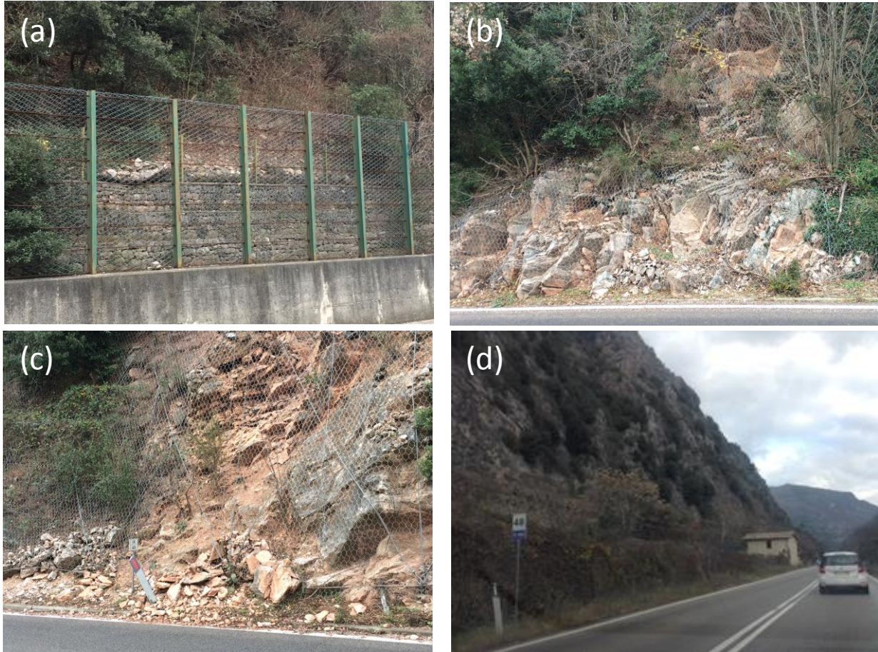
Figure 4.86. Rockfalls between Piedipaterno and Cerreto along highway SS685.
