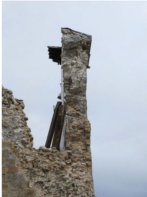
Figure 1. Collapse of the St. Agostino church in Amatrice after the Central Italy earthquake 2016 (image courtesy of the Curia of Rieti).
