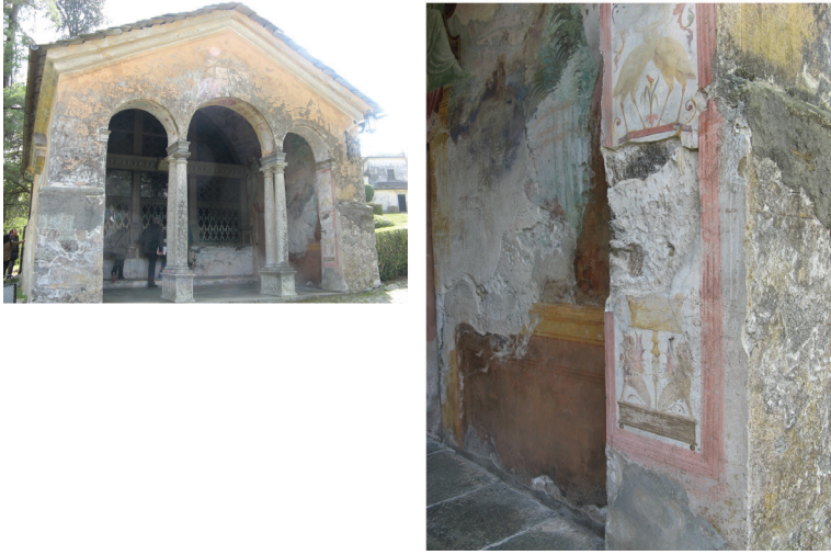
Figure 16. Decay of historical plasters because of the rain infiltrations (Sacro Monte of Varallo).
