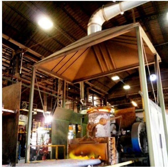
Figure 3. Methane oven in the factory for the heating of steel bars with extractor hood
