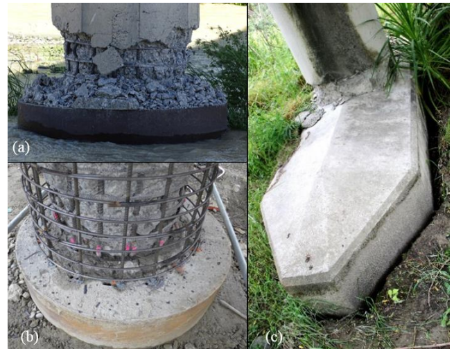
Figure 8. Plastic hinge repair: (a) PH in Lower Mason Bridge; (b) repair of PH by epoxy grout bars; (c) geometry at Mason River Bridge PH zones.
