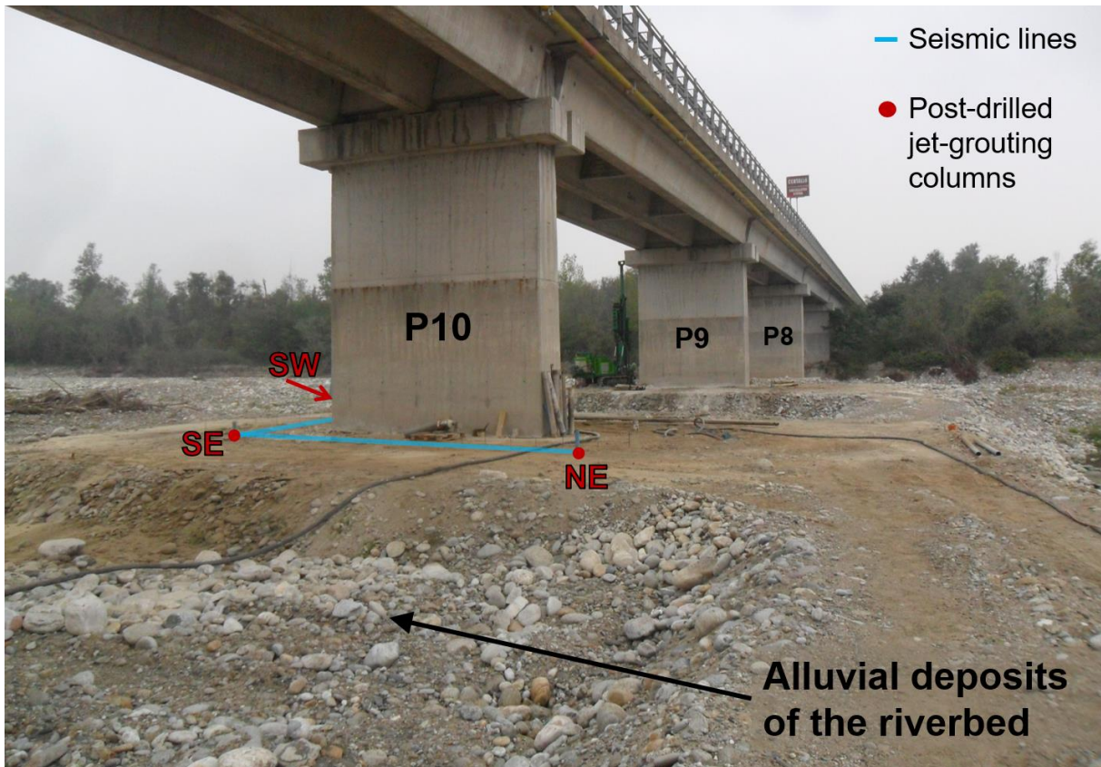
Figure 2 Actual alluvial deposits on the riverbed around the piers of the bridge and completed (P10) or in-progress (P9) jet-grouting interventions on the scoured foundations. Evidences of the post-drilled boreholes used for the surveys and of the imaged seismic sections are also highlighted on P10
