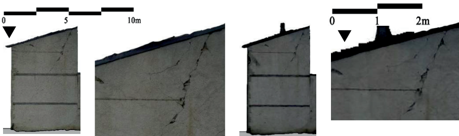
Figure 17. Orthoimage of the East side. The aerial model by integrated oblique and nadir cameras (right), can be comparable in terms of available detail and the accessible information to the terrestrial photogrammetric one (left).
