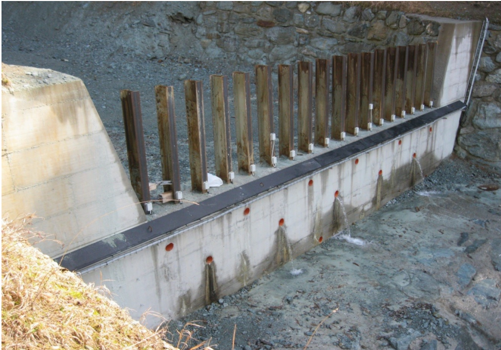
Fig. 7.1 Sectional barrier in Saint-Vincent (Valle d'Aosta Region). It is realised with a 1 m high concrete basement and 2 m high steel piles (IPE 270), spacing 0.5 m from each others. The displacement monitoring system is installed at the base of each piles, downstream the flow. It consists in strain sensors (HBM SLB 700A).
