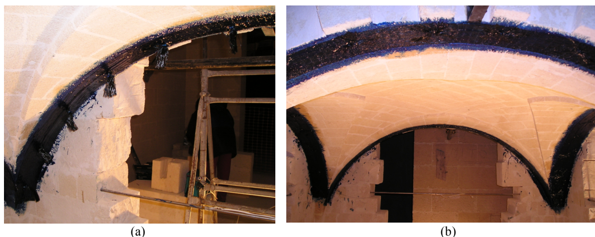
Figure 3 – Strengthening of the vault with FRP sheet. (a) the spikes are inserted through the sheet into the holes; (b) picture of the vault after completion of strengthening.
