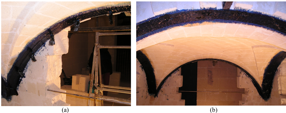
Figure 3 – Strengthening of the vault with FRP sheet. (a) the spikes are inserted through the sheet into the holes; (b) picture of the vault after completion of strengthening.
