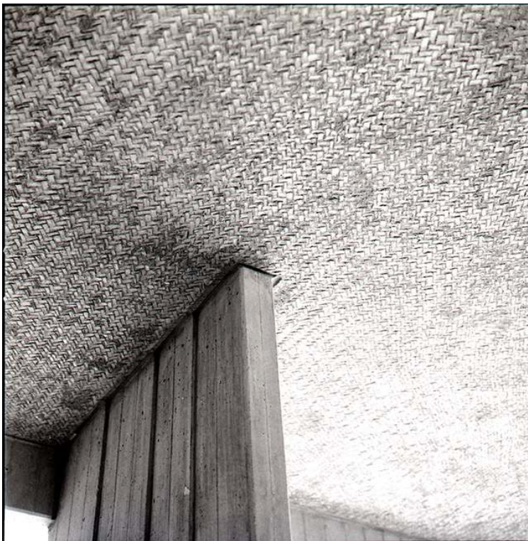
Figure 12: Detail of the mark left by the woven straw mat on the concrete surface.
