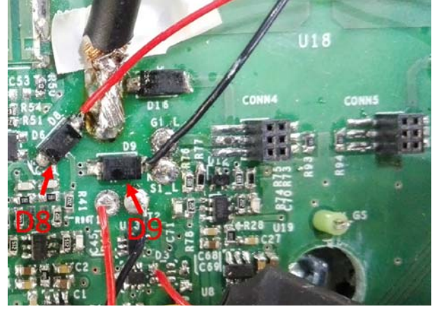
Fig. 6. Detail of the power board. The two diodes D8 and D9 are close to each other.
