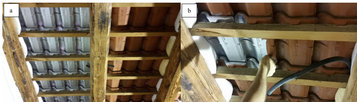
Fig. 3. (a) on the left (config B), on the right (config. A); (b) Low-E treatment by paint brush coating
