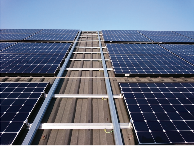
Fig. 3. PV modules, aluminum frameworks and bonding conductors.
