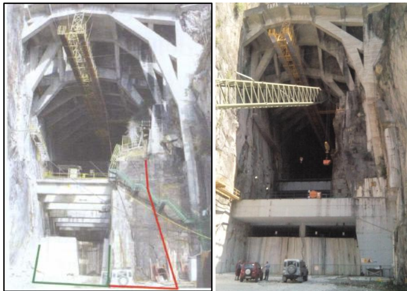
Figure 2. Left: The adit of the Candoglia Cavern before the substitution of the concrete beams and the enlargement on the right side (2000)(Pelizza et al., 2000, 2006). Right: The adit of the Candoglia Cavern after the substitution of the concrete beams and the enlargement on the right side (2014).
