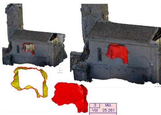
Figure 12. Analysis on West wall where the damage mechanisms caused the collapse of the central part of the masonry by shear failures.
