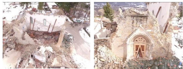
Figure 5. Oblique image of the Sant'Agostino Church; the top of the bell tower and the collapse after the Norcia earthquake; the structure after the January seismic events
