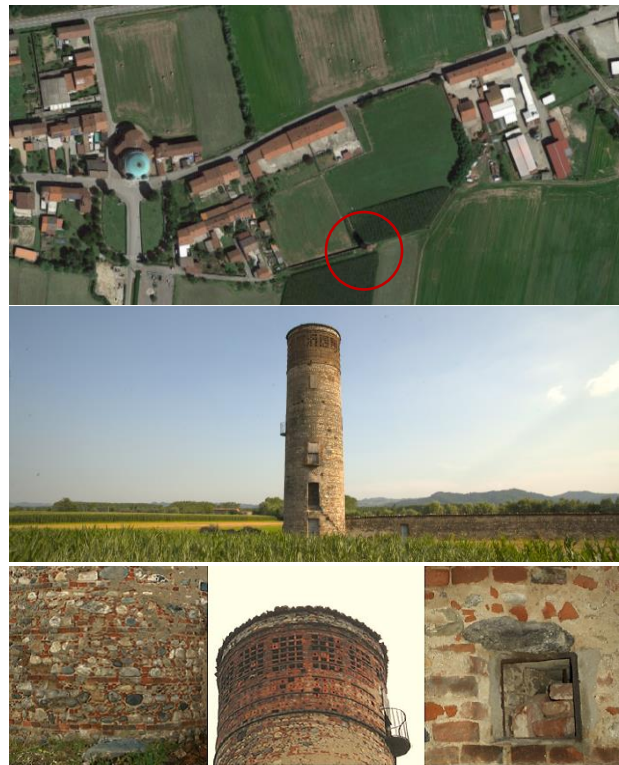
Figure 1. The late-medieval tower. Satellite image by Google©. Details on the dovecot and on mixed stone and brick masonry.
