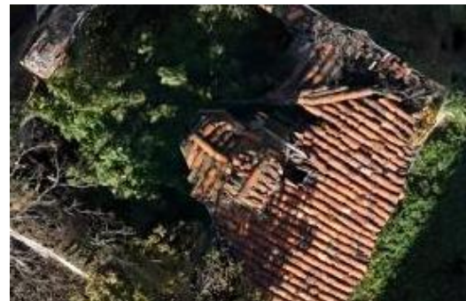
Figure 11. (side column) The 0.212 km 2 extension of the orthophoto covering area, projected on regional DEM. (Nany Matamoros elab.); (above) An excerpt of the 2 cm resolution orthophoto, enabling to examine a collapsed roof.
