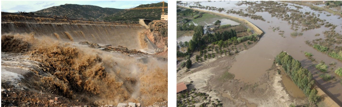
Figure 2 The Maccheronis dam (left) and a portion of the embankment (right) after the flood event.
