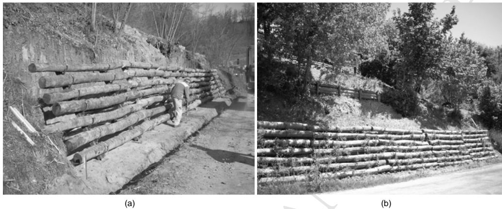
Fig. 4. Example of the structure installed at Roatto (Asti, Italy): (a) the element before the filling, and (b) final configuration when the bushes start growing.
