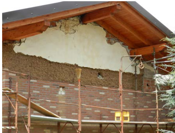
Fig. 3. Application of an external coating on an earthen building in san Giuliano Nuovo, (Alessandria, Italy).
