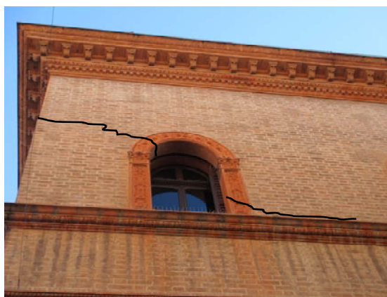
Fig. 4 Diagonal cracks on external windows
