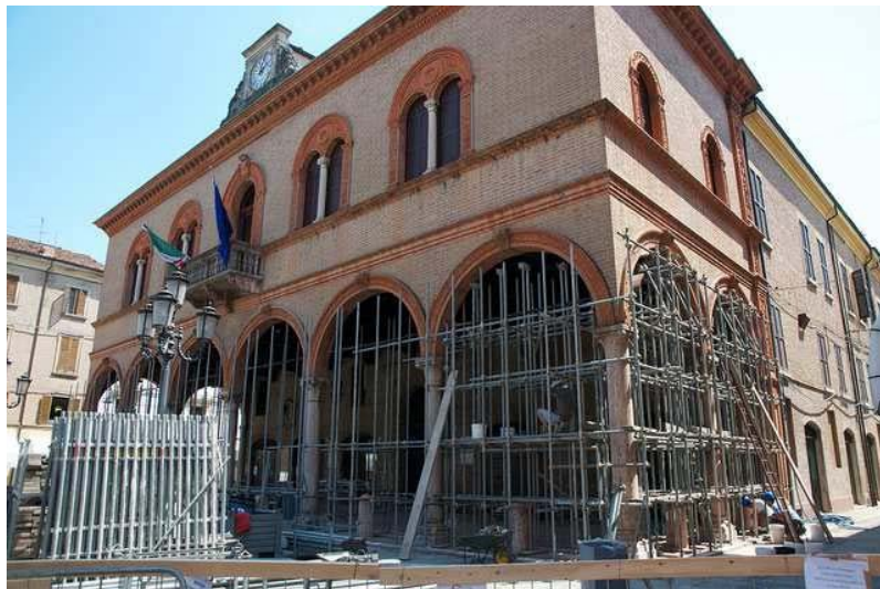
Fig. 13 Scaffolding in the North-West side of the Facade during May 29 th Shock
