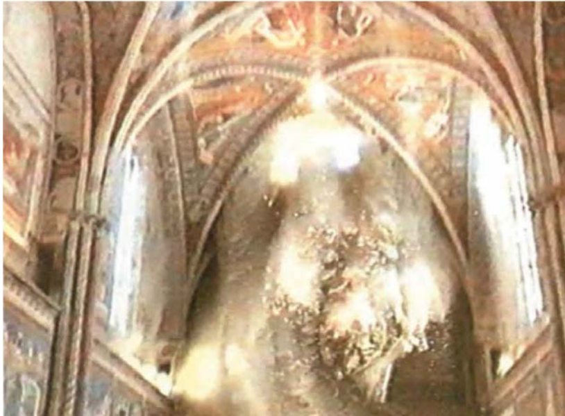
Figure 4- Collapse of the vault of the Doctors of the Church (Bonsanti, 1998).
