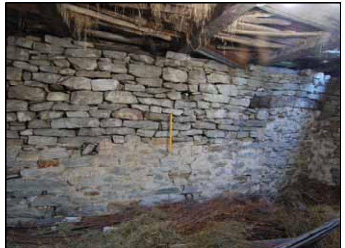
Fig. 2. Interior stone wall of an Alpine traditional building (located in Veglio, hamlet of Montecrestese, Italy)
