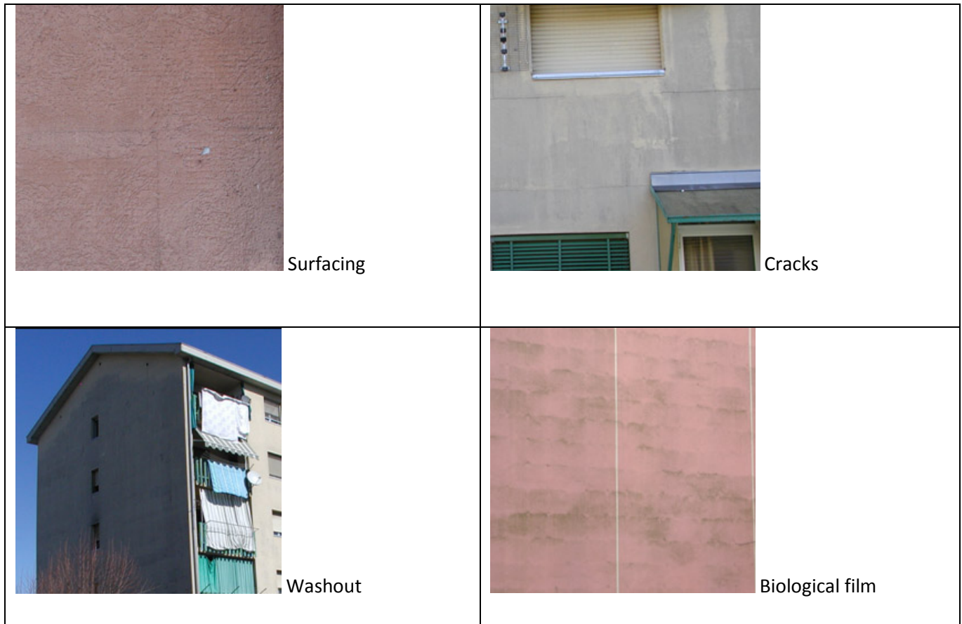
Fig 2: The main defects considered in the study.
