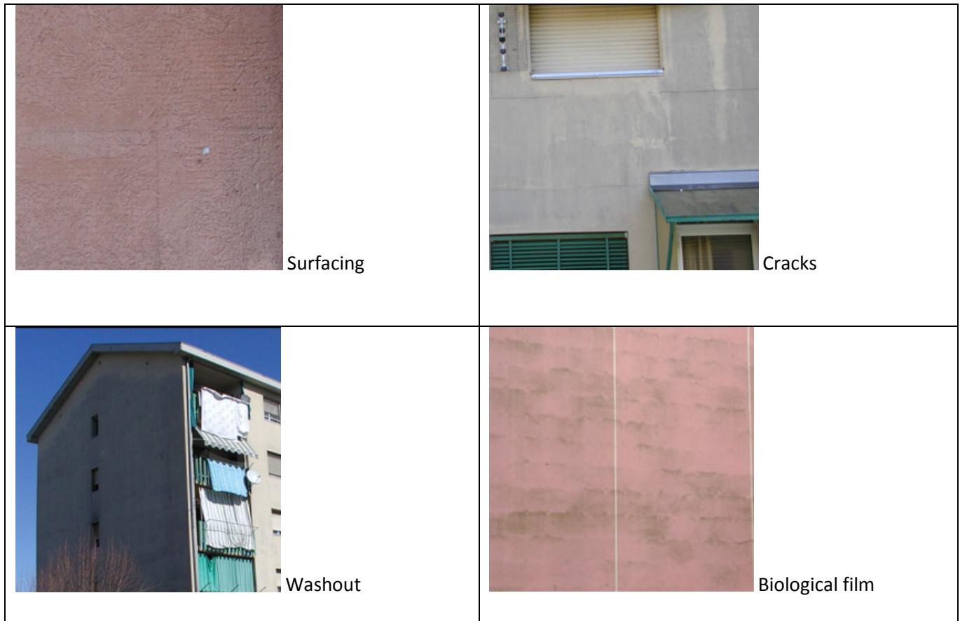
Fig 2: The main defects considered in the study.
