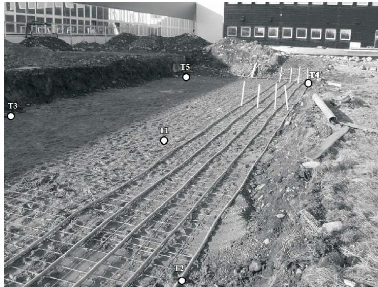
Fig. 3. View of the pipes and position of the thermometers.
