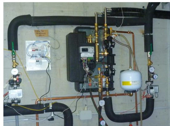
Figure 5 –FPC Pumping and heat transfer station
