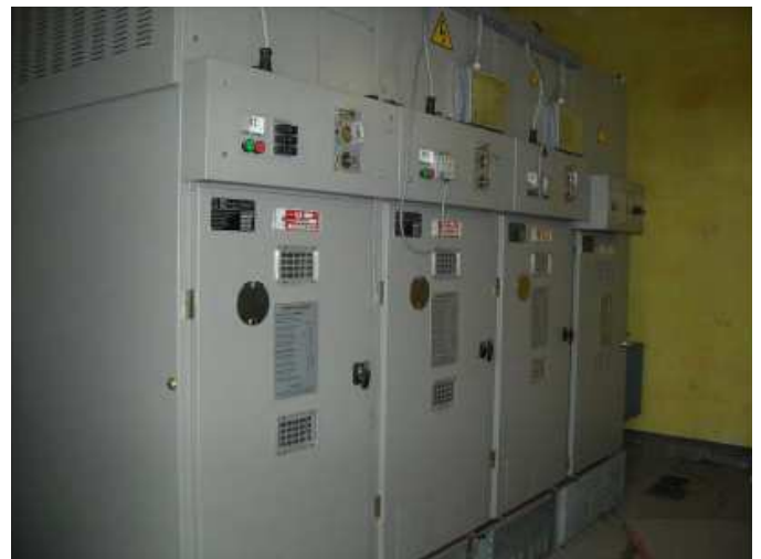
Fig. 5. MV switchgear in the faulted substation.
