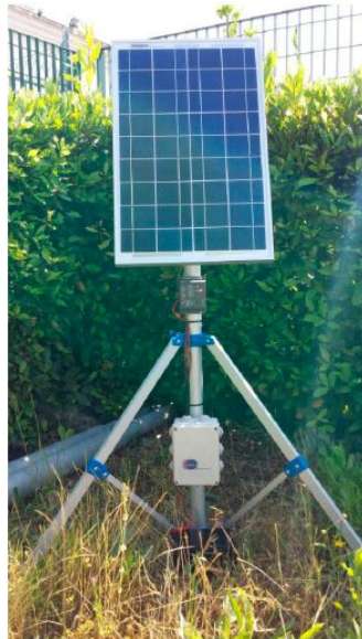
Figure 29. One of the nodes (enclosed in the white box) with its solar panel.
