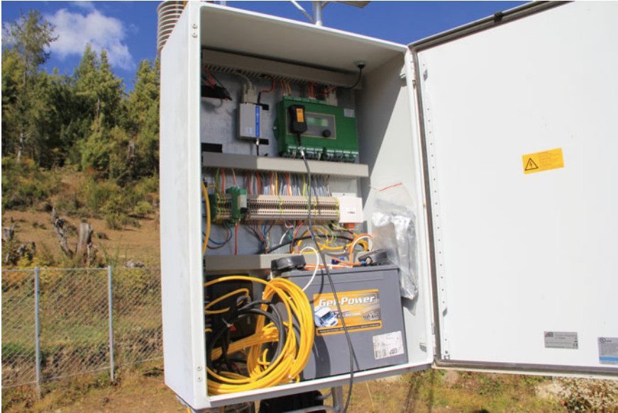
Fig. 2.3 Rara Nepal. OTT data logger and data transmission modem in IP65 enclosure
