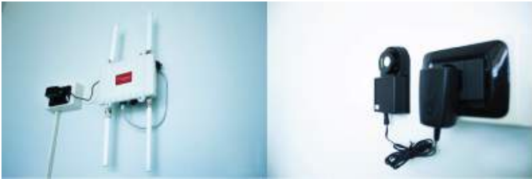
Fig. 31 Crowd-sensor (left) and temperature, humidity and CO 2 sensor (right) installed in the out-loud study room at CLE
