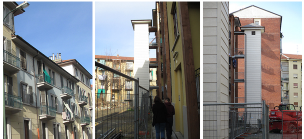
Figure 2 –the context: inconvenience and degradation due to the construction yard
