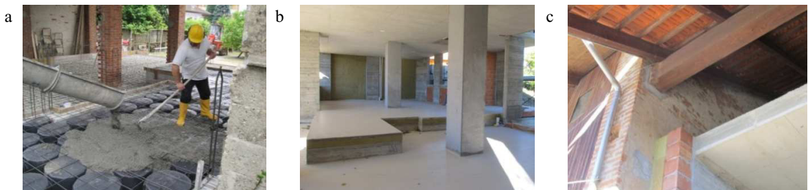
Fig. 2. (a) casting of the floor slab above disposable formworks; (b) structure of the house with insulation layers; (c) roof details.
