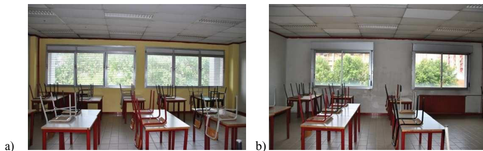
Fig. 3. Daylighting systems for classrooms at 1 st floor (a) and 2 nd floor (b)
