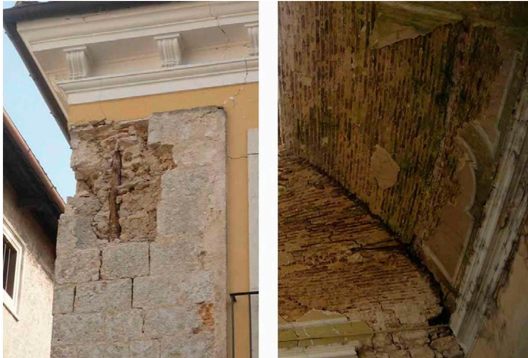
Fig. 2. L'Aquila: vertical wooden log, probably part of a more complex wooden frame (on the left). L'Aquila: wooden tie-rods in a cloister vault in Palazzo Ardinghelli (on the right).
