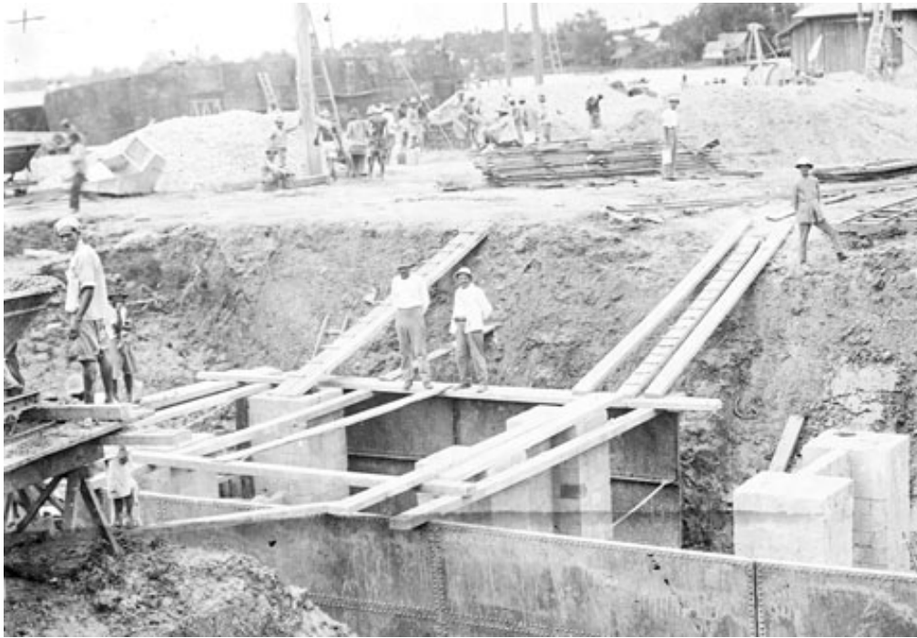
Figure 9: Chests of metal prepared for the foundations of the piers of the Memorial bridge.
