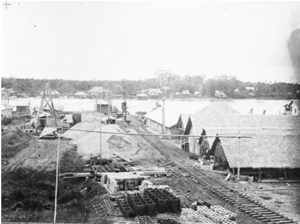
Figure 6: Works along the banks of the river for the site preparation for the construction of the Memorial Bridge at Bangkok, Thailand.
