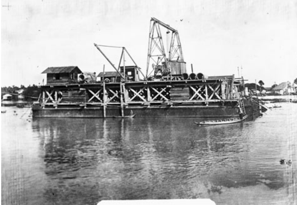
Figure 5: Excavations and pipe laying foundations for compressed air in the Menam Chow Phja River at Bangkok, Thailand.
