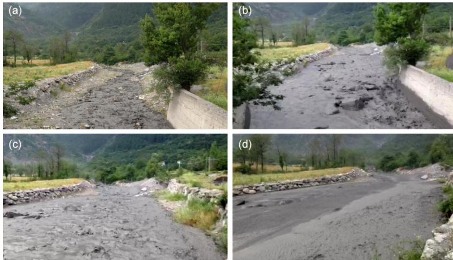
Figure 28 - Frames of the video recording made by an inhabitant of the village of Novalesa along the Malo torrent, few meters upstream the confluence with the Cenischia stream, on July 17, 2013. All view are from downstream to upstream: (a) the channel bed few minutes before the arrival of the main front; (b) the debris flow boulder front; (c) a secondary liquid surge; (d) the muddy tail of the phenomenon.
