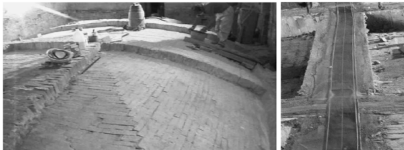
Figure 1. (a) The masonry vault and reinforcement arches dated 1600 during surface preparation for CFRP application. (b) Smart CFRP sheet placed on vault [3].
