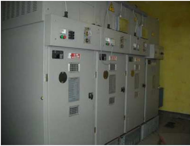
Fig. 6. MV switchgear in the faulted substation.
