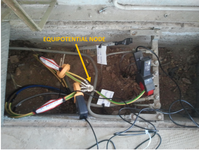
Fig. 5. Equipotential node in the MV/LV substations
