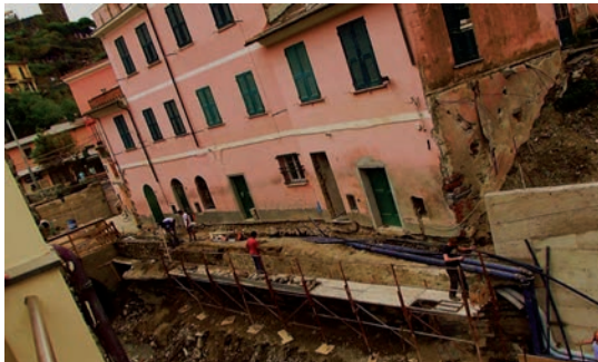
Figure 2.a Flood damages in July 2012.
