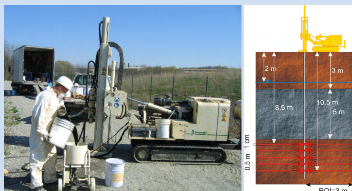
Field injection via direct push (courtesy of Carsico S.r.l., left) and scheme of stratigraphy and injection points (right)
