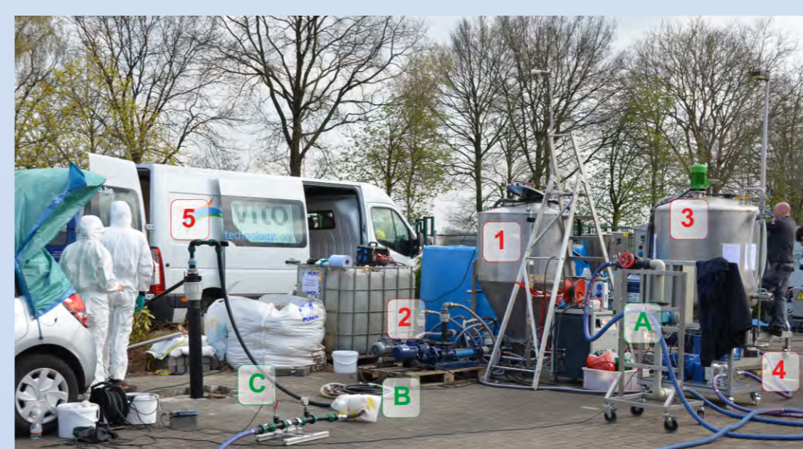
IMZVI field injection at Site P: (1) tank for slurry preparation (2) dispersion and recirculation unit, (3) tank for slurry storage, (4) cation pump, (5) injection well, (A) discharge rate measurement, (B) magnetic susceptibility sensor, (C) pressure sensor.
