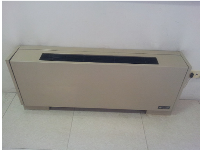
Fig. 3. Example of fan coil unit under examination
