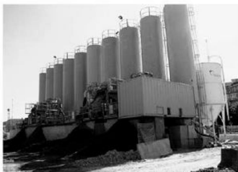
Fig. 4 Compact slurry treatment plant (dewatering, fines separation and partial bentonite recycle) installed for Turin Railway "Passante" works (Oggeri, 2009).
