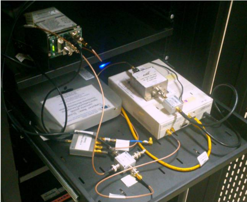
Figure 2. Hardware installed at Hanoi for collection of GNSS scintillating signals.
