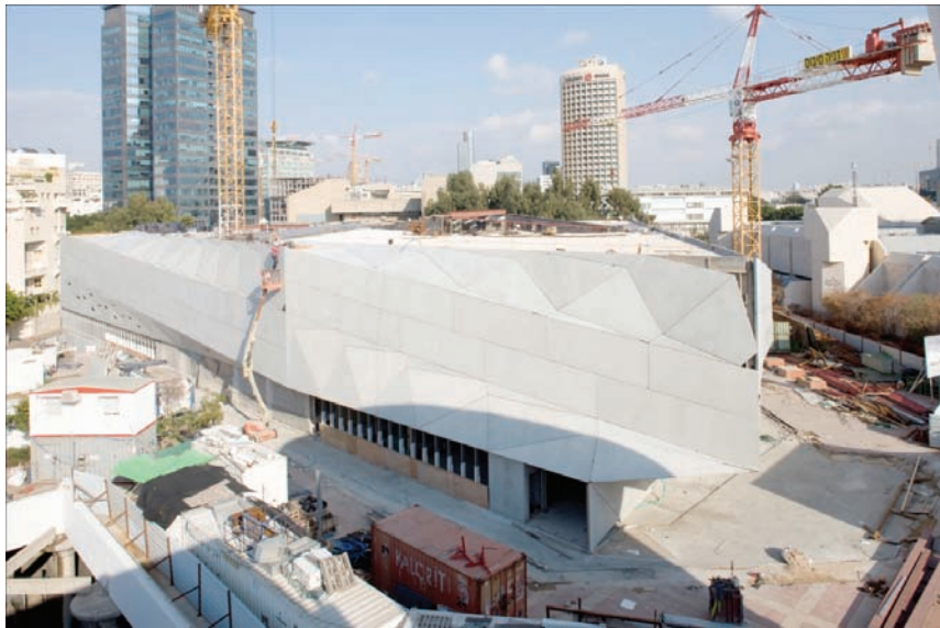
Figure 2. Overview of the construction site of the Tel Aviv Museum, showcasing the assembly of the concrete panel façade. Source: The Tel Aviv Museum of Art.
