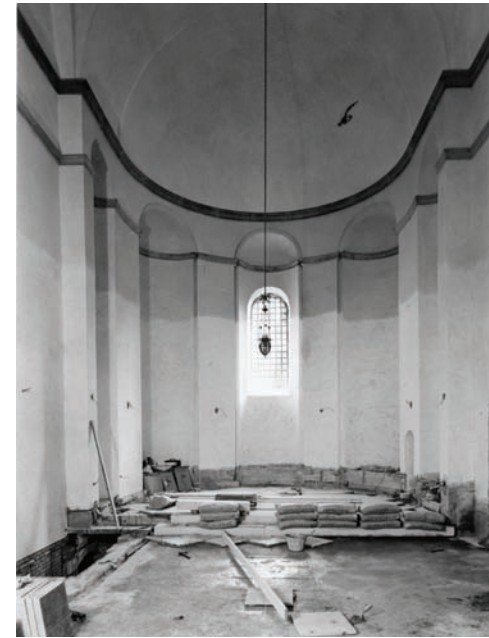
Figure 1. Chapel of San Teodoro: interior view during the 1961 restoration, when its original appearance was restored. Source: Archivio Procuratoria di San Marco.
