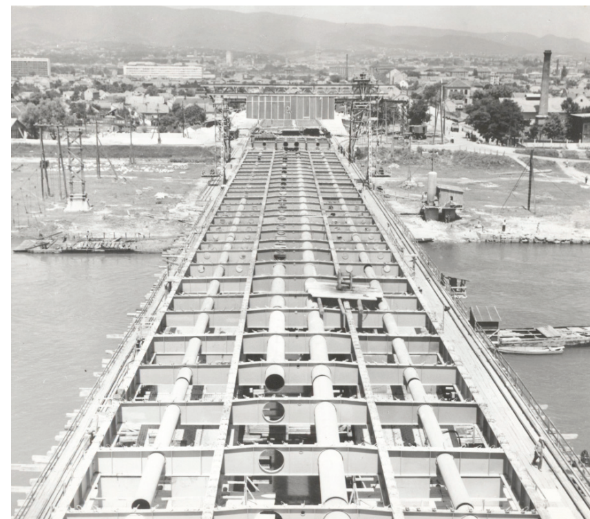
Figure 1. The Bridge of Freedom under construction in the early 1950s, enabling the city's expansion southwards and the later construction of modernist city of Novi Zagreb. Source: HR-MGZ-PA [41.310], 1958, Milan Pavić
