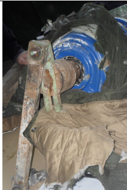
Figure 38 evident traces of the original placement of the connecting rod - crank axis of the gearbox bolted into place with tilt and less eccentric crank
